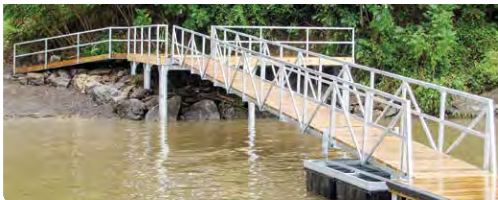
Above Top: T-shaped steel truss floating dock system. Above: Our shoreside platform as the shore anchor.
