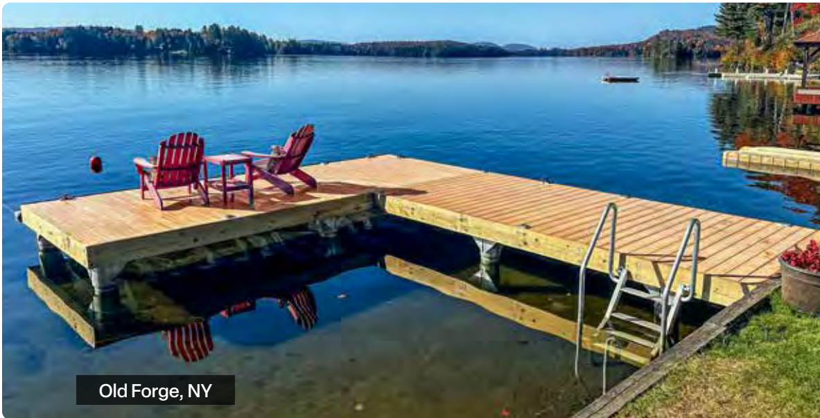
Below: L-shaped pile dock with Weardeck decking and our shallow water stairs.
