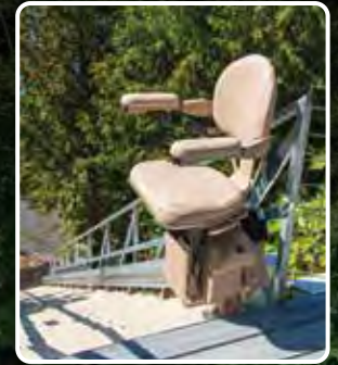
Custom stair designed with added width and structural components to accommodate a stair lift chair (installed by others)
